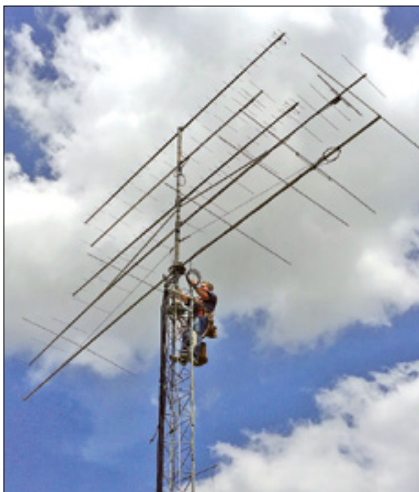
Figure 1 — This doesn't look like the "lower" four bands, but George, K5TR, can be seen hard at work getting his VHF/UHF array ready for the contest. From bottom to top (not including George) are seven elements on 50 MHz, 17 elements on 144 MHz, 16 elements on 222 MHz, and a pair of 28-element beams on 432 MHz. [George, K5TR, photo]
