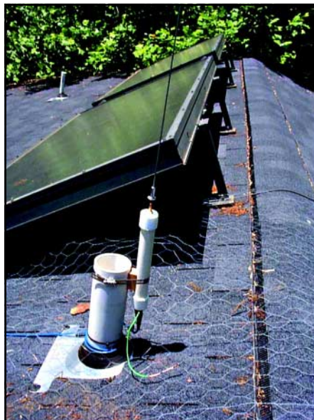
A sheet of chicken-wire screening can be laid beneath the antenna and connected to the antenna ground to stabilize the fields around the antenna to further reduce noise coupling. Chicken-wire screening in rooftop installations is generally hard to see from the ground.
