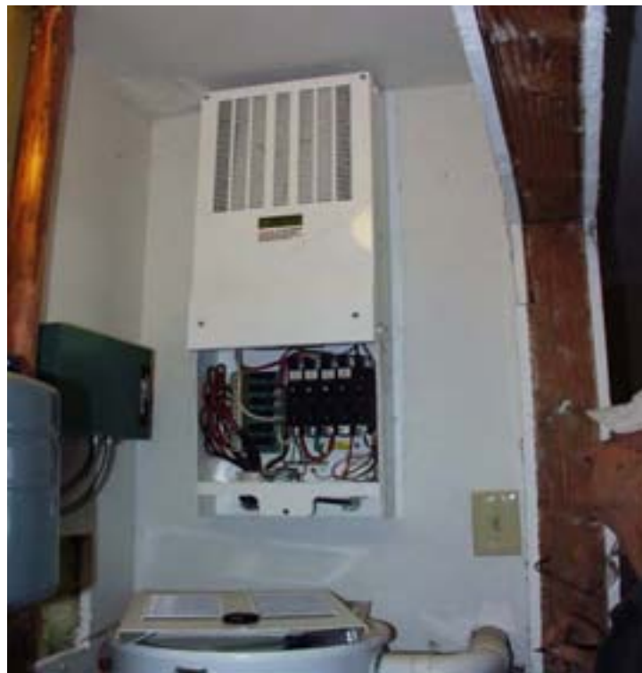
Figure 51 Solar Power Converter
