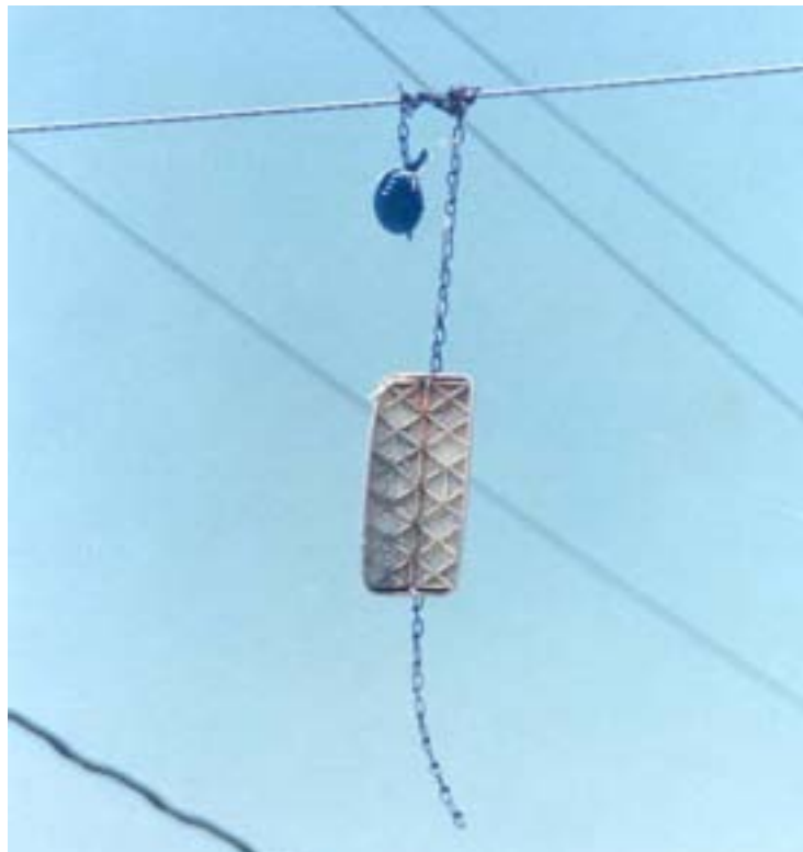
Figure 44 Debris on a Distribution Line Conductor
