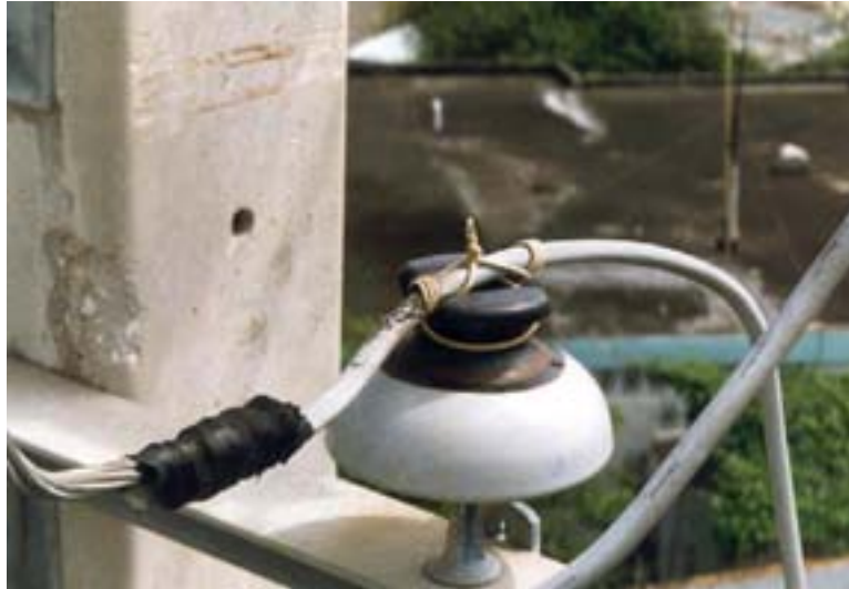
Figure 35 Insulated Tie Wire on an Insulated Conductor
