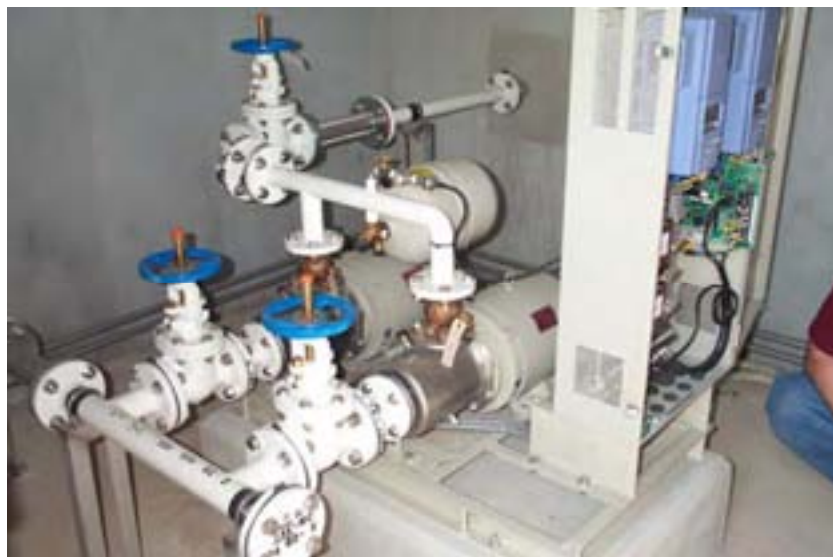
Figure 50 View of Variable-Speed Motors and their Loads
