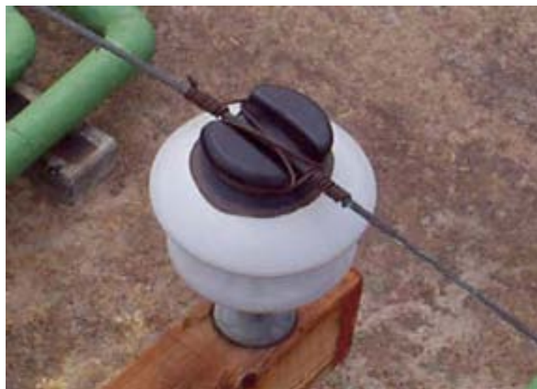
Figure 36 Insulated Tie Wire on a Bare Conductor
