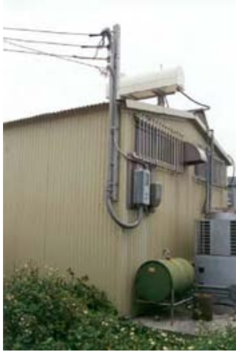
Figure 53 Power Feed for Hydroponics Farm
