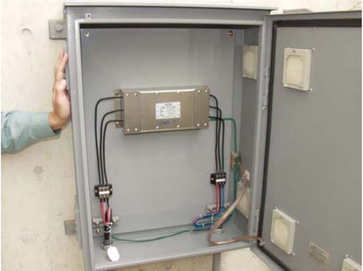
Figure 75 Improper Filter Configuration
