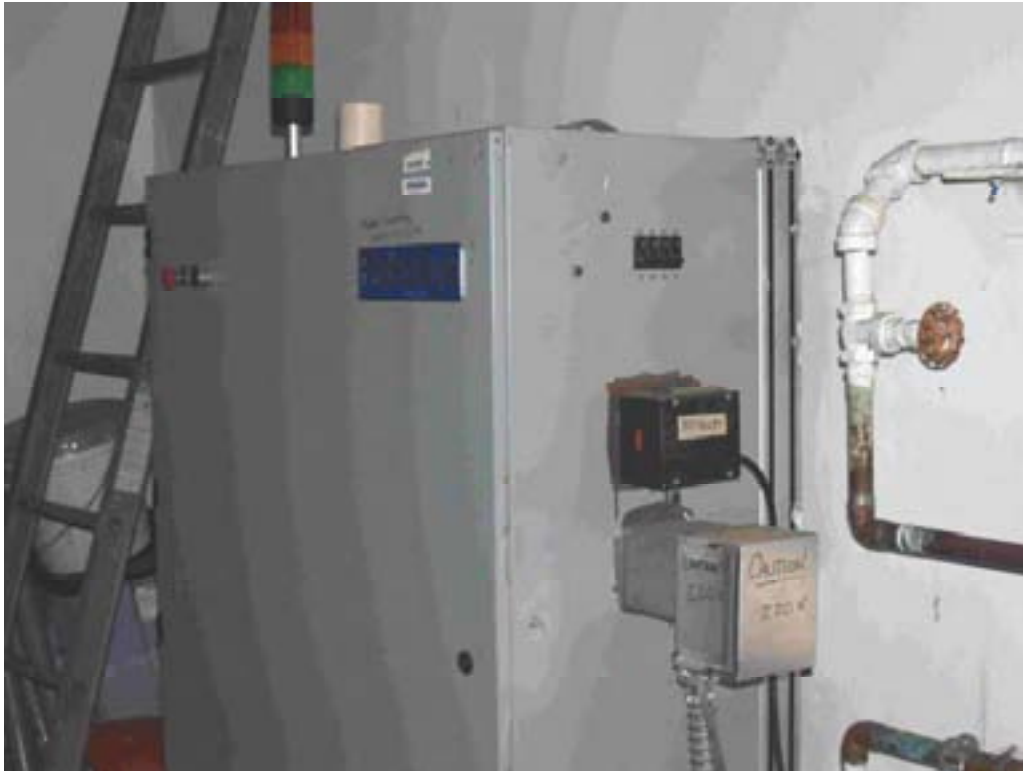
Figure 74 Filter Installation to Suppress Motor-Controller Noise
