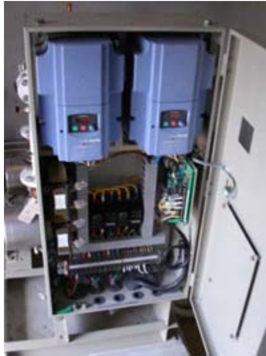
Figure 49 Variable-Frequency Controllers for Two Electric Motors
