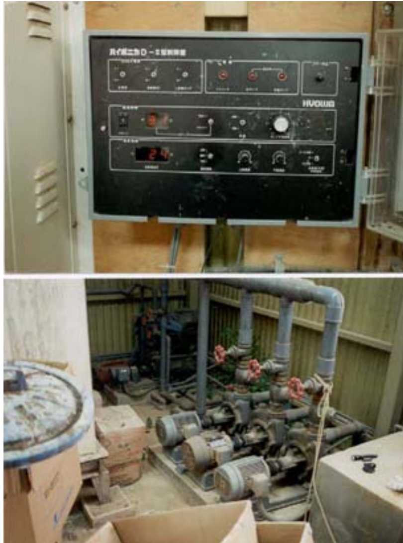
Figure 52 Motor Controller at a Hydroponics Farm
