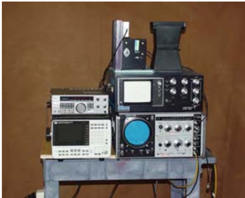
Figure 6 Photograph of Typical Site Instrumentation
