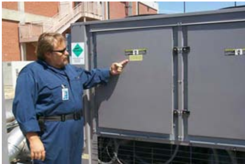
Figure 48 Housing for Variable-Speed Motor Controller and Motor
